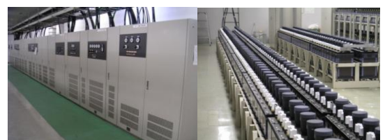
無停電電源装置(UPS) ※UPS: Uninterruptible Power Supply
