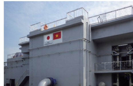
U-BCF* being constructed at An Duong Water Treatment Plant (Hai Phong City)
