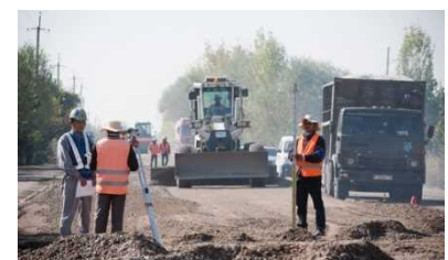
(Photo) OJT for formwork and road paving on-site (Courtesy of Dai Nippon Construction)
