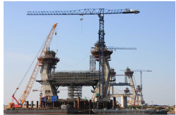
(Photo) Main tower construction with self-ascending/descending work platforms (Courtesy of Sumitomo Mitsui Construction)
