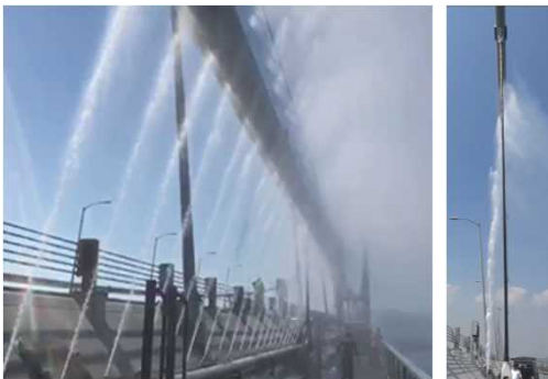
(Photo) Water cooling system
