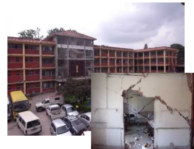
(Photo) Overview of the stricken Paropakar Maternity Hospital (upper photo) and the hospital interior (lower photo) (Courtesy of K.I.T.O Architects & Engineers)
